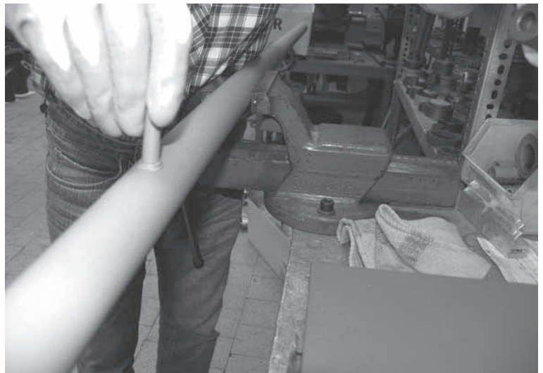
Fig. 2 Remove the welding device and insert the repairing plug precisely without twisting it.
